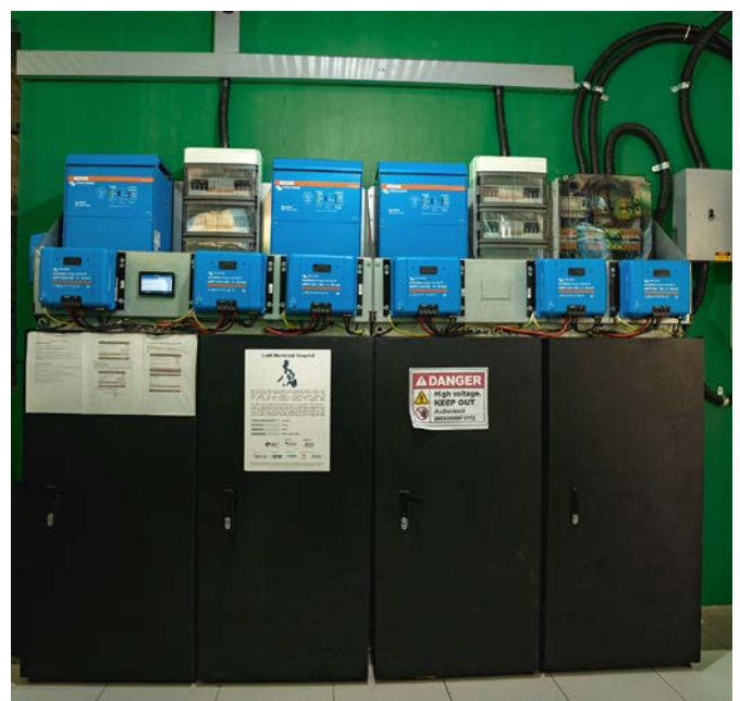
The battery and inverter system in the installation
