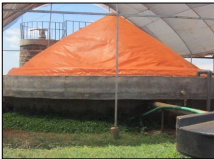
Figure 15: Biogas plant at Simbi Roses
