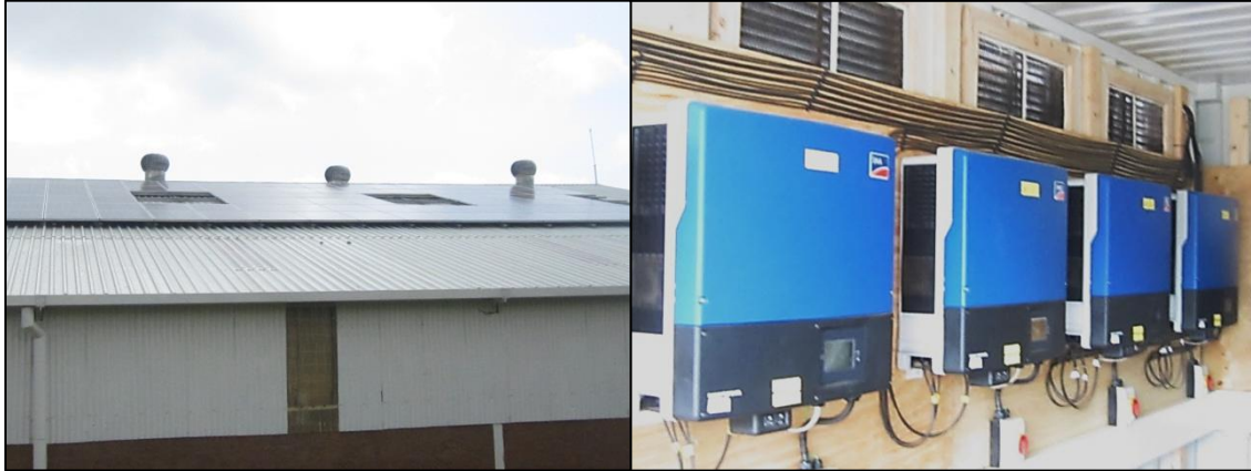
Figure 7: Roof-mounted PV installation & inverter installation at Uhuru Flowers
