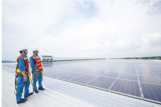
308 kW p system, the first for local cold chain
