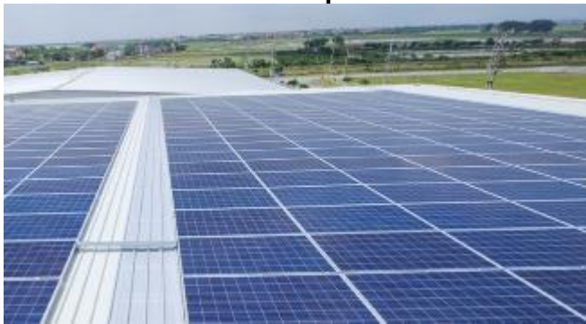
Emergent cold, Vietnam – 308 kWp
