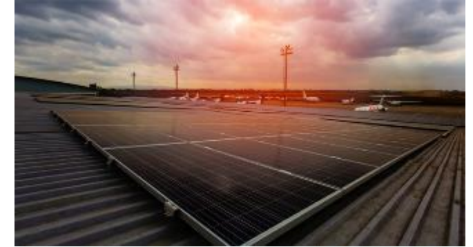
Swissport Kenya Limited, Kenya – 110 kWp
