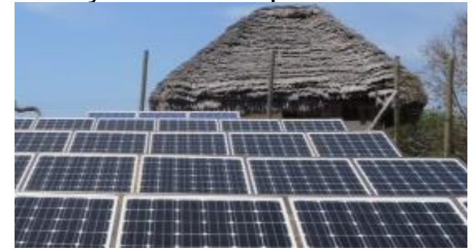
Travessia Lodge, Mozambique – 10 kWp
