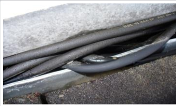
Example 1: Pinched cables due to incorrect installation
