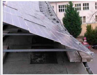
Example 2: Moving PV system due to insufficient weight on mounting structure
