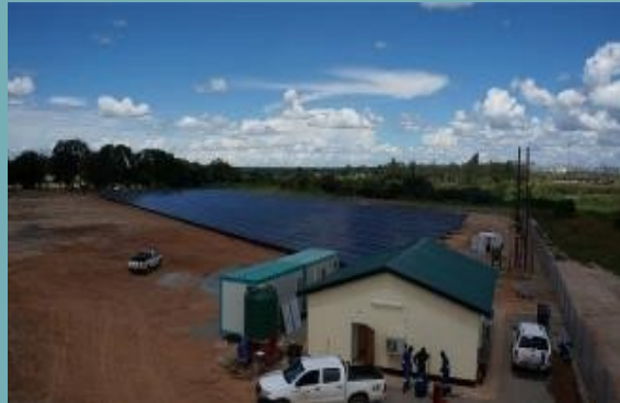
Copperbelt Energy Corporation, Zambia 1 MWp
