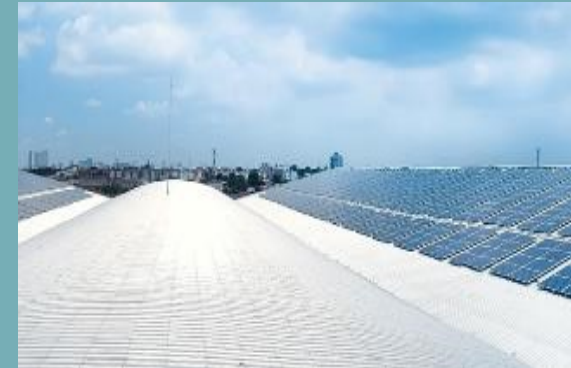
Star Aire, Thailand 1 MWp
