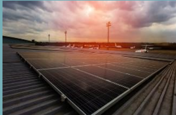
Swissport Kenya Limited, Kenya 110 kWp
