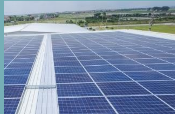
Emergent cold, Vietnam 308 kWp
