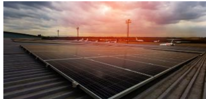
Swissport Kenya Limited, Kenya 110 kWp
