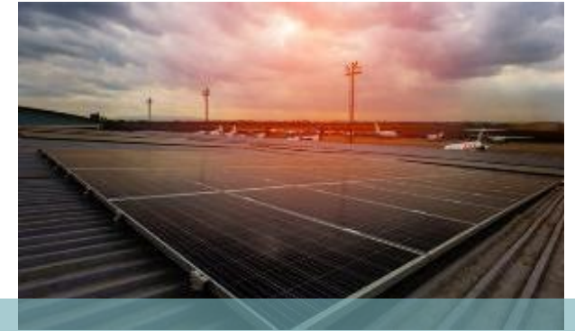
Swissport Kenya Limited Kenia, 110 kWp © Light in Captivity / Stephen
