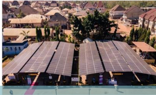
NCDC Lab Nigeria, 260kWp & 500kWh storage
