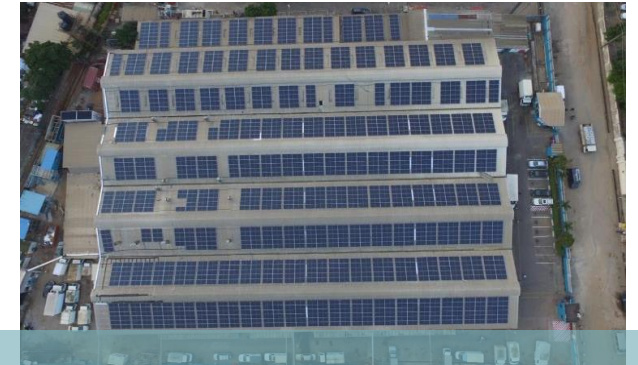
UAC Dairies Nigeria, 800 kWp
