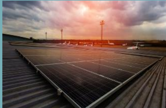
Swissport Kenya Limited, Kenya 110 kWp
