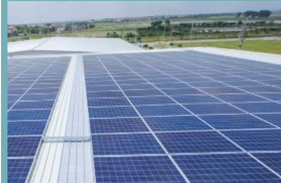
Emergent cold, Vietnam 308 kWp
