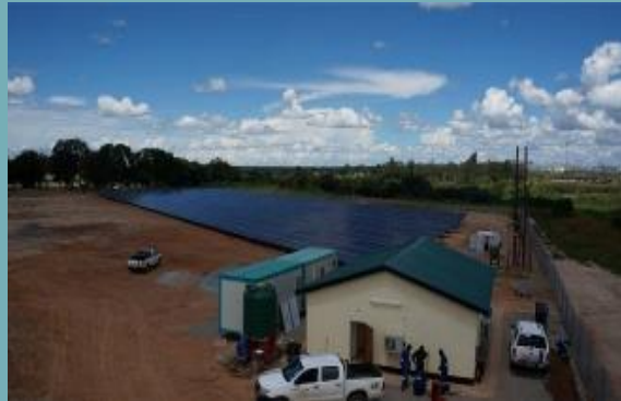
Copperbelt Energy Corporation, Zambia 1 MWp
